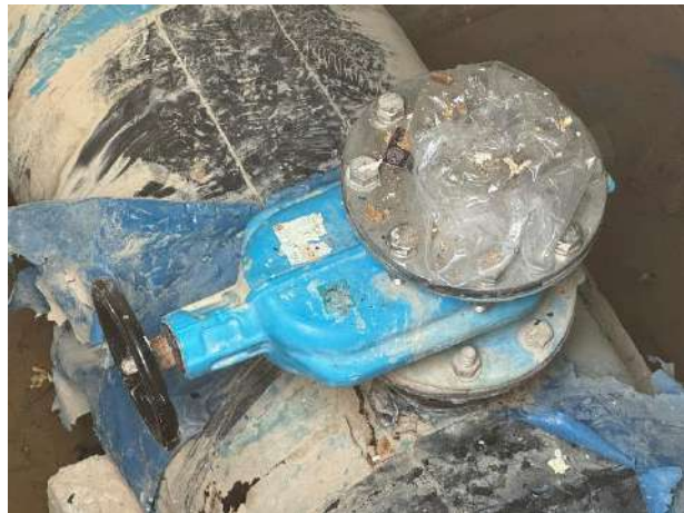
Gate valve entry point
